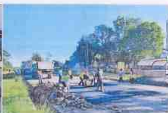
Tarmac Patching along Lunatic Road, Nanyuki Ward
